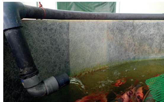
Retorno de agua al recipiente / Water return to the tanks
